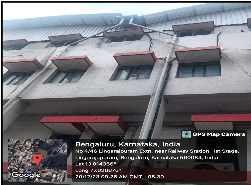
Image of the Rainwater harvesting provision
